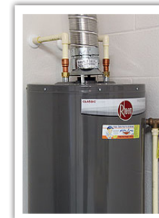
50 Gallon Gas Water Heater
