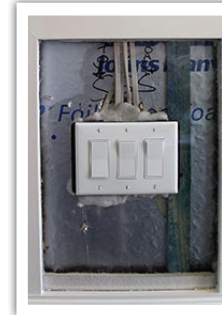
Insulated Electrical Outlets
