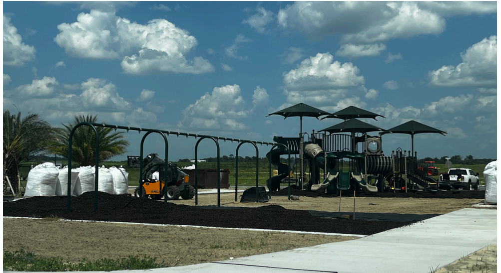
Playground equipment was installed at Adventure Park in Sorrel Glen in late August.
